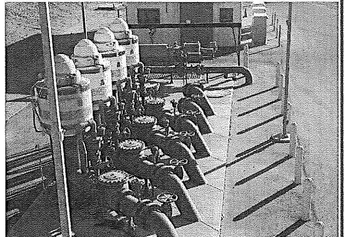
OH Booster Plant and variable frequency drive.
